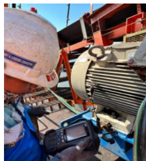
Figure 8. Inspection data Motor and Gearbox using tools
