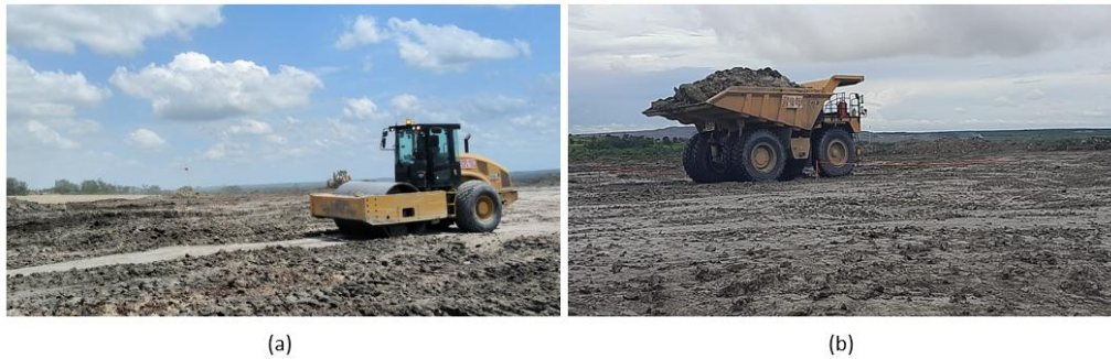
Figure 12. (a) Compaction test with Compactor Cat CS79 and (b) Compaction test with heavy dump truck HD Cat 777
